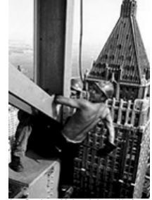
Joe Regis, a Mohawk Iron Worker, erecting the Chase Manhattan Building -1960, NYC
